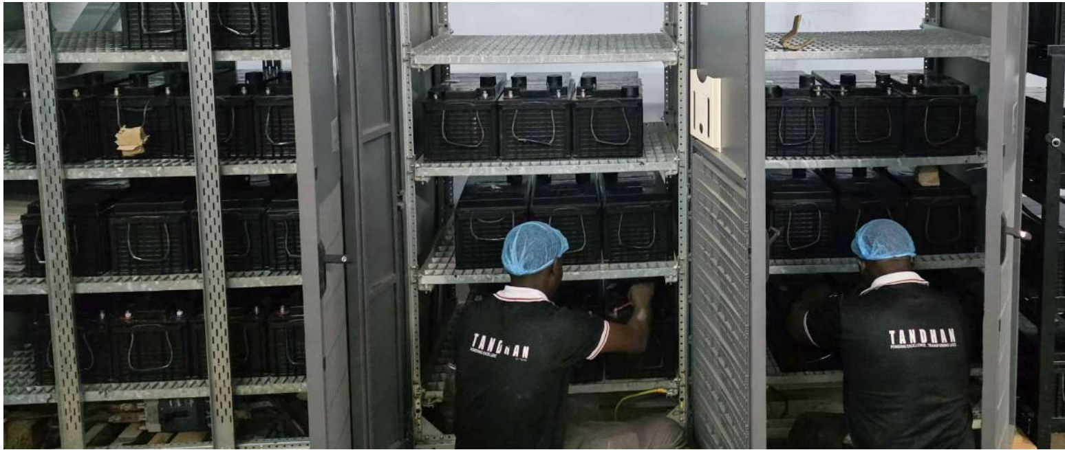
DPI 500KVA UPS Battery replacement using Tandhan Power NXT VRLA SMF batteries at Digital Packaging Innovations Holdings Ltd, a state-of-the-art printing facility in Kenya.
