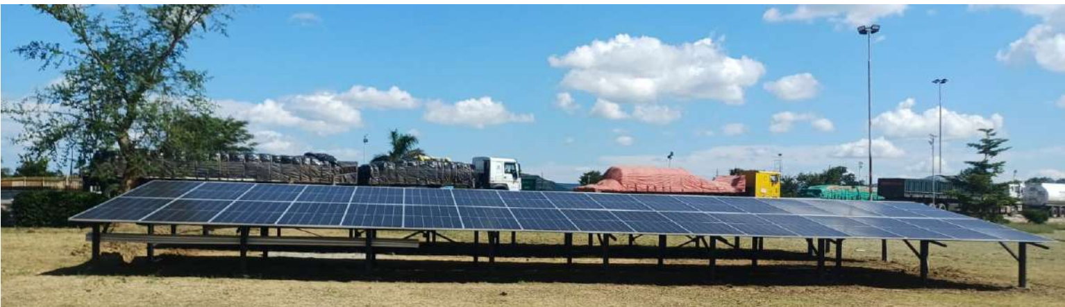
50kW solar system with 183.6KWh battery storage system commissioned at RDA weighbridge Kafue Zambia
